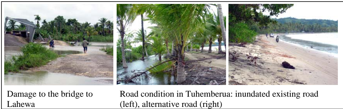
Figure 3. Condition of Infrastructures in Nias Island (photo: Yuliana C. Wulan)
