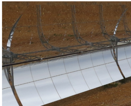
Figure 3. Solar collector element (SCE) with 28 mirrors and three absorber pipes.
