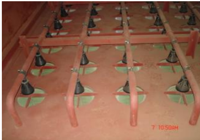
Figure4.8: The inlet air filters
