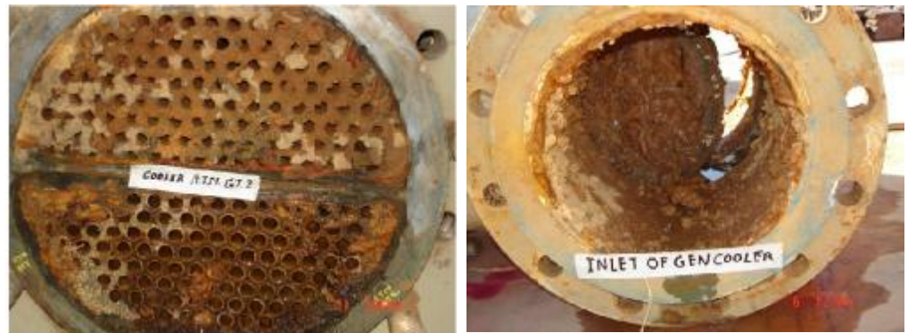
Figure 4.4: fouling of generator cooling system
