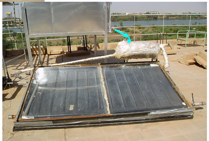
Fig. 4.5 Flow of Rich Ammonia Solution to Flat Plate Collector (smaller storage capacity) at Sunshine.
