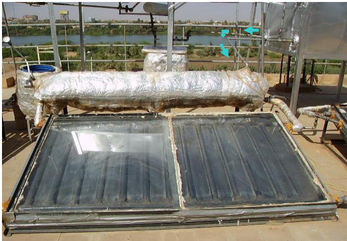
Fig.4.4 Flow of Rich Ammonia from Absorber to Flat Plate Collectors (greater storage capacity) at sun shine.
