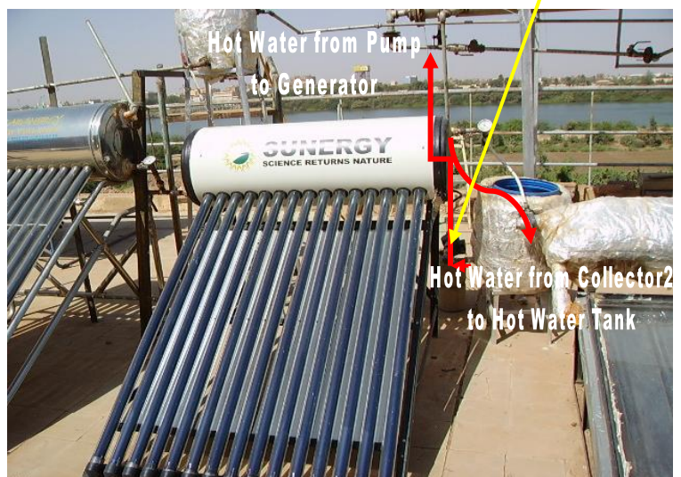
Fig. 4.27 Hot Water Pumping from Storage to Generator
