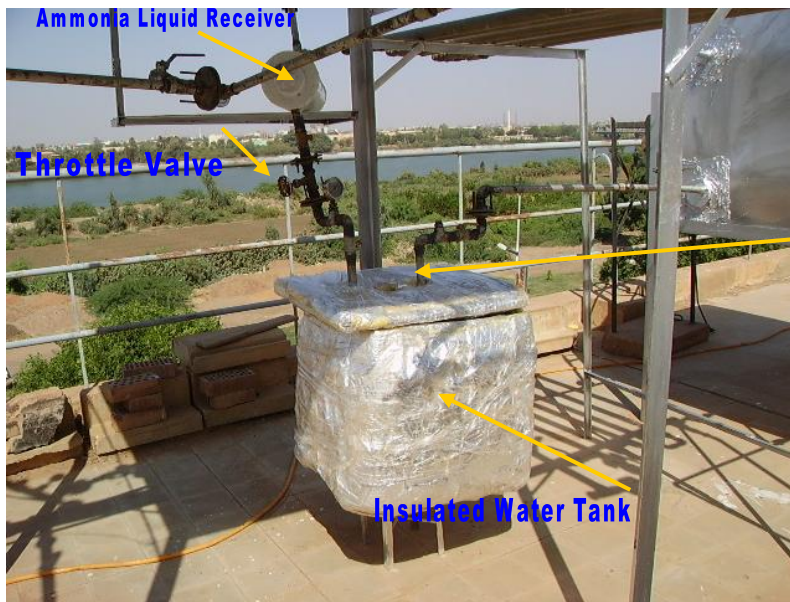
Fig.4.18 Evaporator coil in the insulated water Tank
