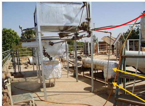
Fig. 4.35 Mixing of Hot Water with cold Water to Obtain Water with Different Temperature
