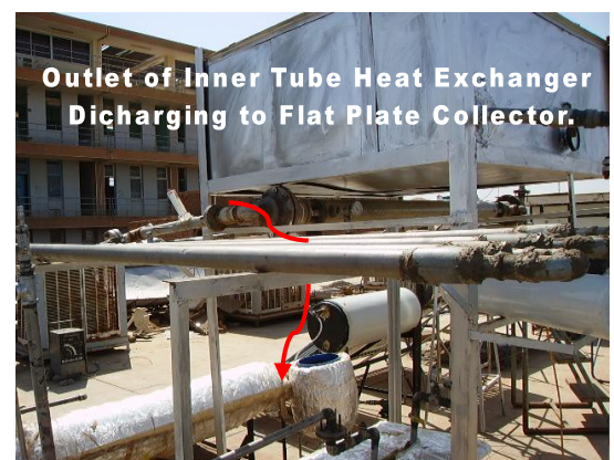
Fig. 4.32 Connection of Outlet of Inner Tube of Double Heat Exchanger to Flat Plate Collector
