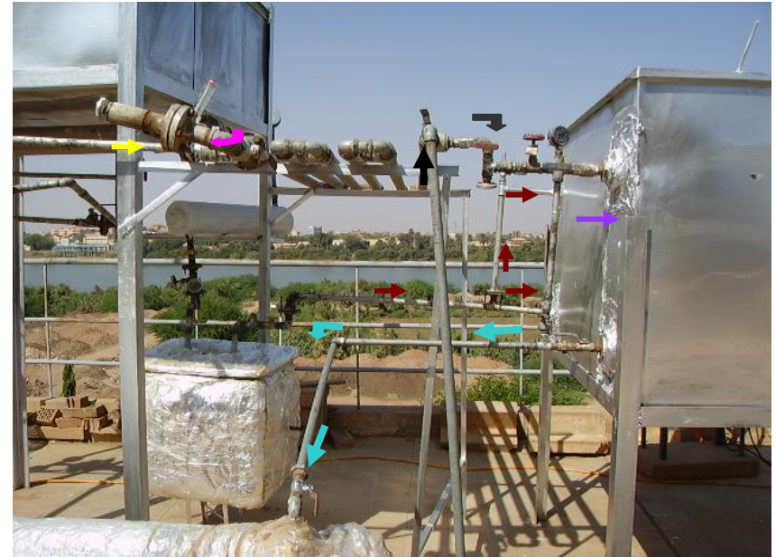
Fig. 4.7 Flow of Rich & Poor Ammonia Solutions to and from Solution Heat Exchanger and Absorber.
