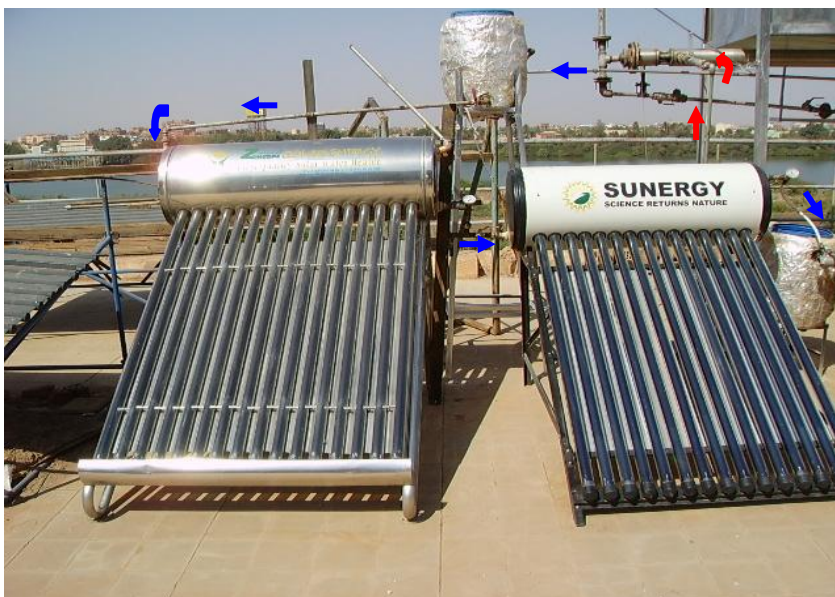
Fig.4.8 Circulation of Hot Water from Evacuated Collector to Generator and back to Collector.
