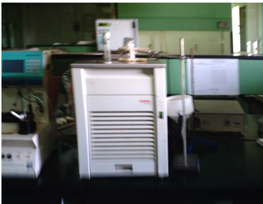
Photograph. B.4: Chiller
