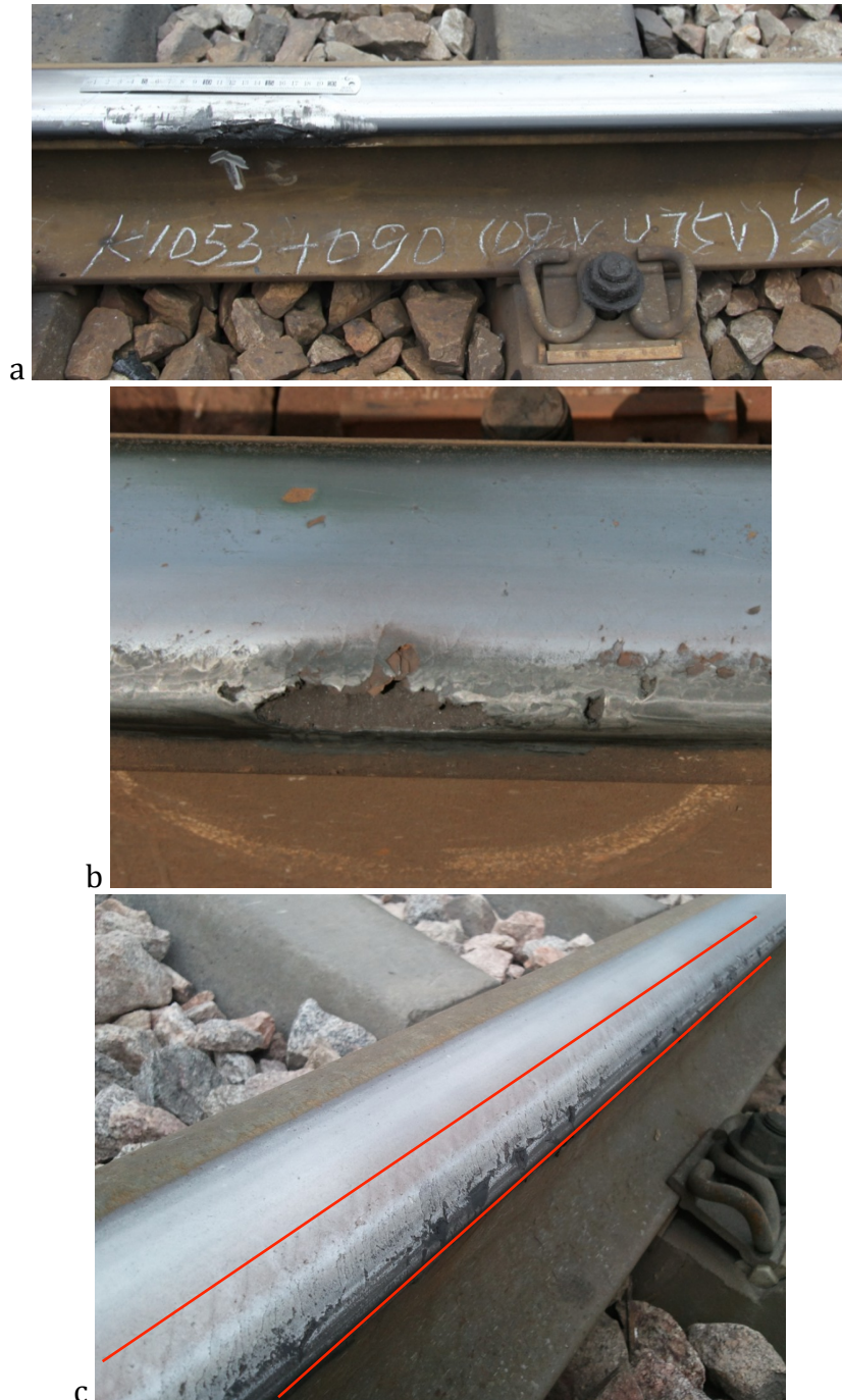
Figure 1 Rail damage corresponding to the cases reported above a) shelling caused by incorrect super-elevation causing cant excess; b) shelling caused by excessive lubrication in order to reduce the lateral wear c) head checks and shelling caused by the use of as-rolled rail, which is not a suitable choice for the current conditions.
