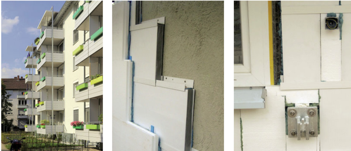
Figure 1. VIP used in the retrofitting of a multi-family building in Karlsruhe, Germany. The 40 mm thick VIP was attached to the façade in a rail system and covered on the exterior by 50 mm EPS. The aim of the design was to maximize the surface covered by VIP (Photo: Schöck Balkonsysteme GmbH, Brillux GmbH & Co. KG).
