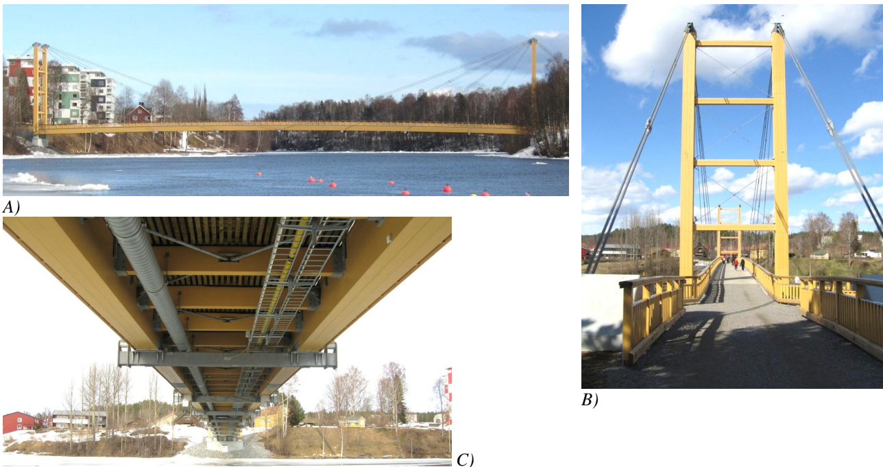
Fig. 2 A) Overview of the bridge, B) The south pylon of Älvsbacka Bridge with its anchorage cables and concrete foundations, C) The main beams are supported by steel cross-beams to which the cables are attached.
