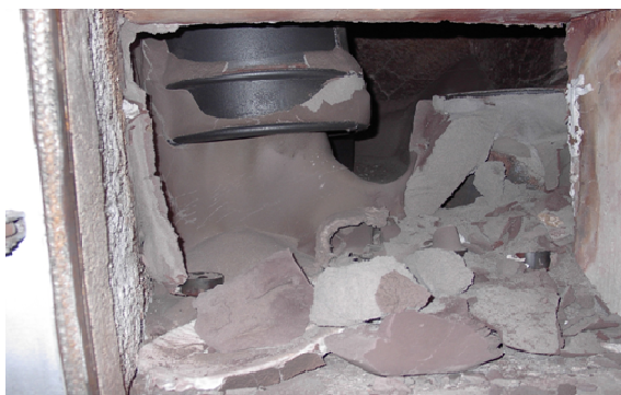
Fig. 2.1. Agglomeration in the loop seal of a CFB boiler after operation with a fuel mix of 20% straw.
