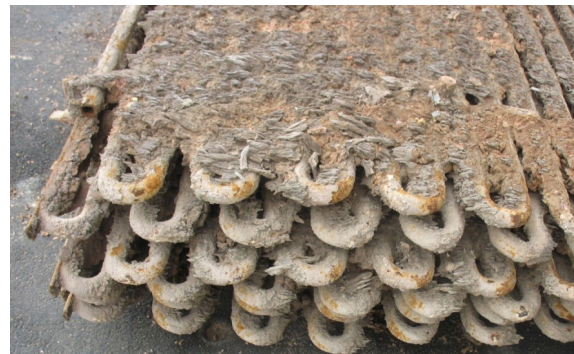
Fig. 2.2. Deposit formation on a superheater used in a grate fired boiler during combustion of waste wood.
