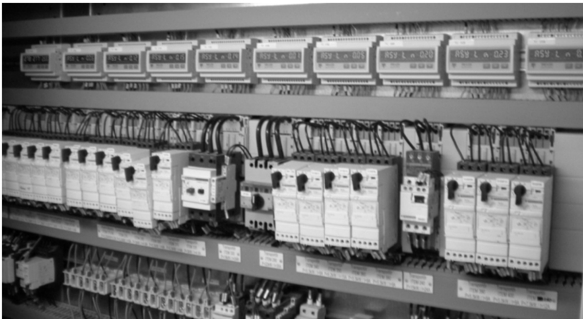
Figure 25. Inside an electrical cabinet on one of the test plants. In the top of this figure, ten power meters can be seen.
