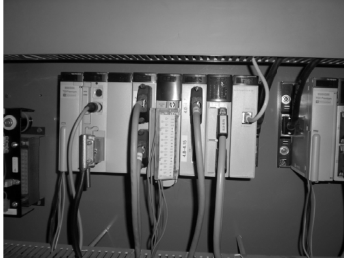
Figure 26. A rack-based PLC from Schneider. The PLC is divided into a CPU, analog and digital IO-modules, and communication modules.
