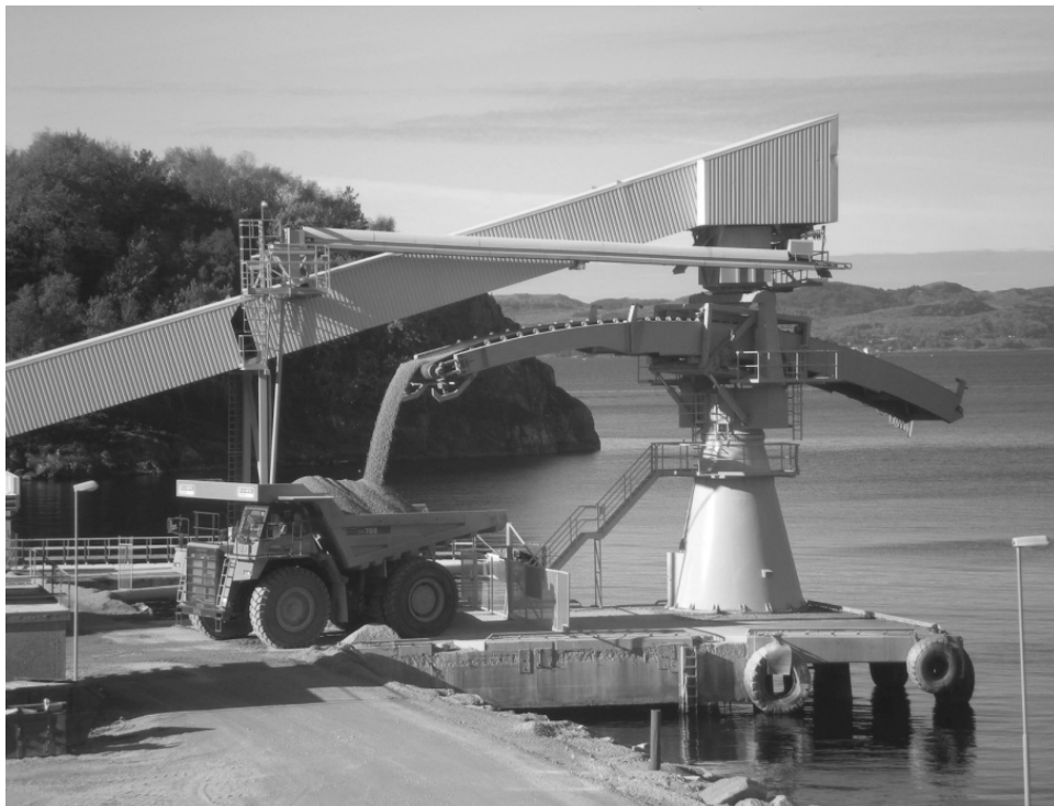
Figure 4. Loading equipment on the quay that can be used for ships and trucks. Norstone AS' Tau plant, Norway.
