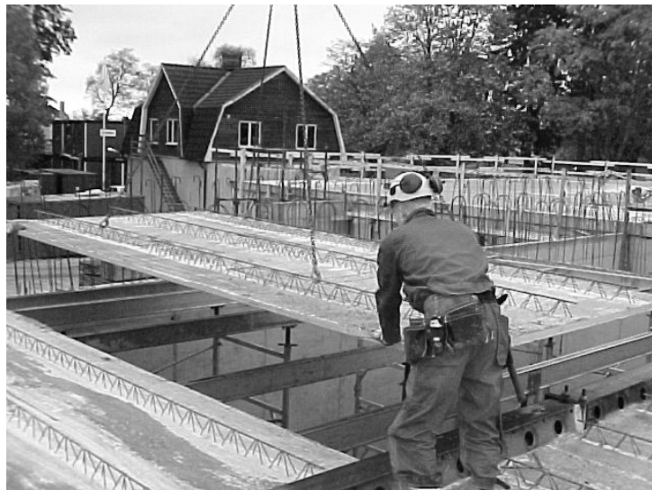
Figure 1. Mounting of lattice girder elements on the construction site (photo, Hans Olsson SKANSKA, Mellerud).
