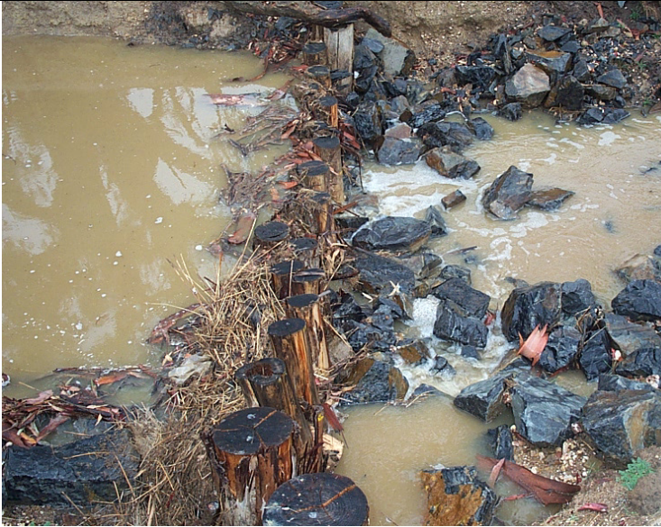
Porous Weir Sediment Trap formed by Driving Timbers into the Creek Bed
