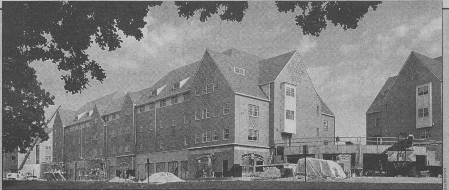
Nearing completion Work on the South 40's new residential houses continues on schedule. Workers are relocating the walkway between the ball fields, landscaping and installing a brick patio. A clock tower will stand at the intersection of Shepley Drive and the walkway, serving as a focal point. The project will be completed in August.
