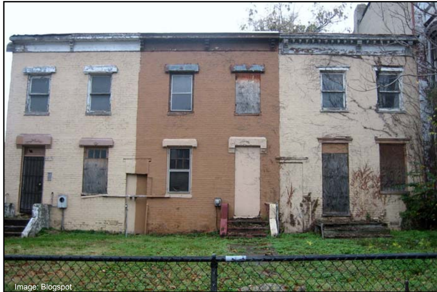
Image 2: Troubled properties can negatively impact the surrounding community fabric
