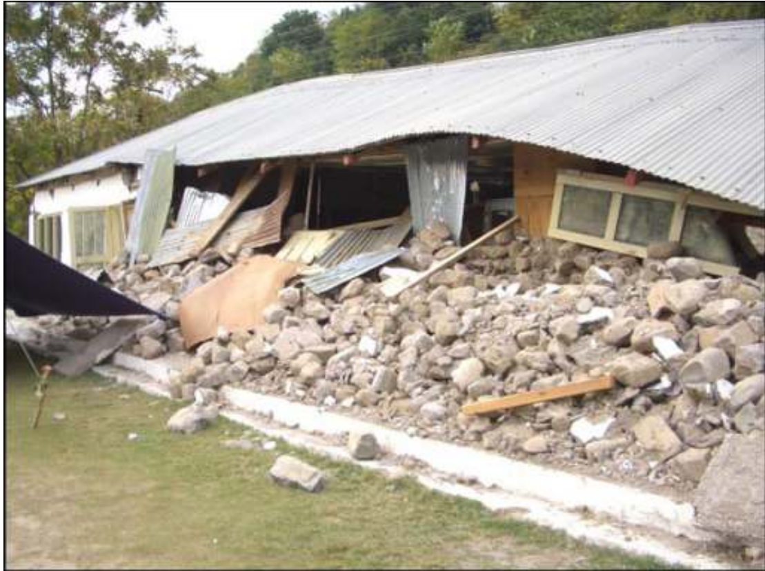
Figure 7: Collapsed Stone Masonry Building
