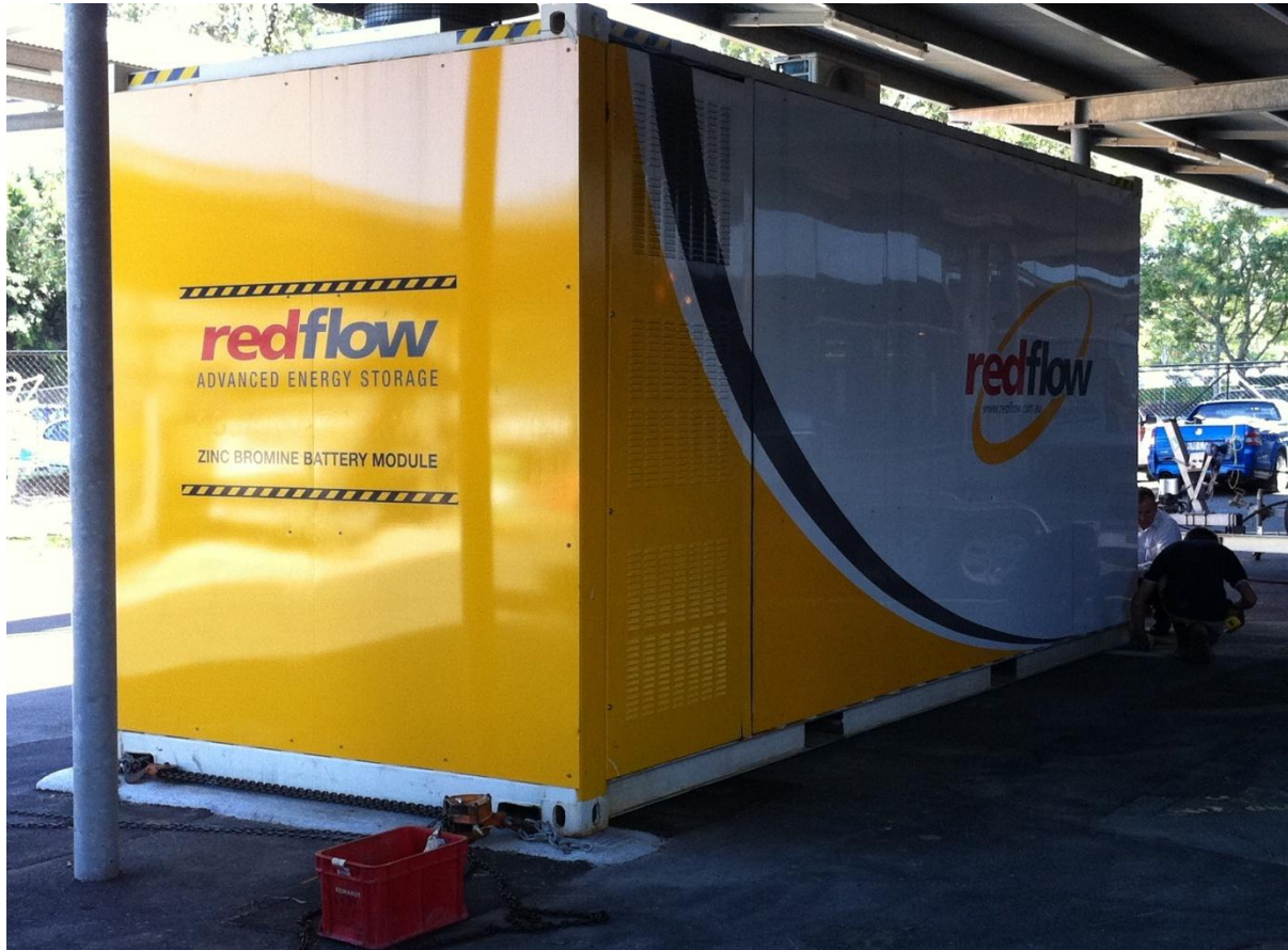
Figure 4 - RedFlow Battery (April 2011)
