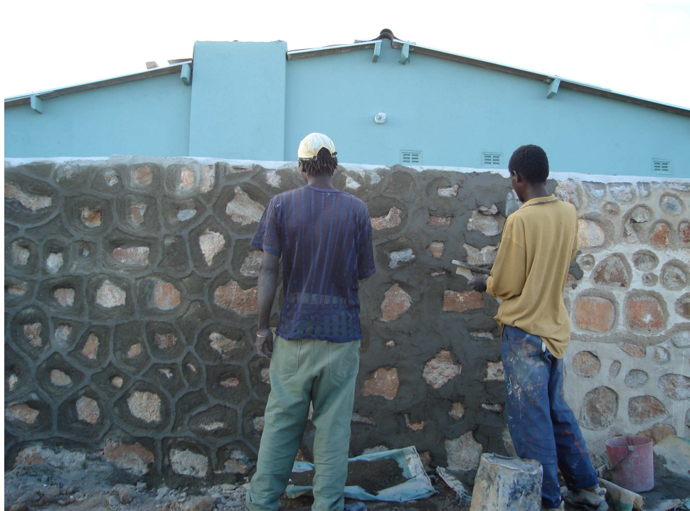
Plate 1: Informal sector builders putting up a masonry wall. One of the many Injiva driven activities in Pumula South. © Mbiba, April 2006.
