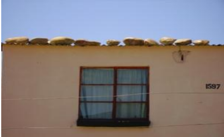
Figure 3: Unsecured Roofing. Hankey, Eastern Cape. Source: Khanya-aicdd, 2008: 10.
