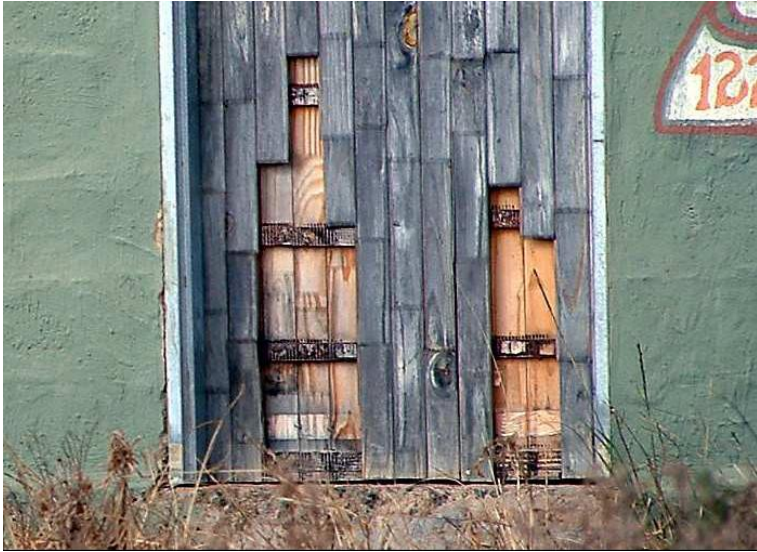
Figure 6: Broken Door. Peddie, Eastern Cape. Source: de Nobrega, 2007: 12.
