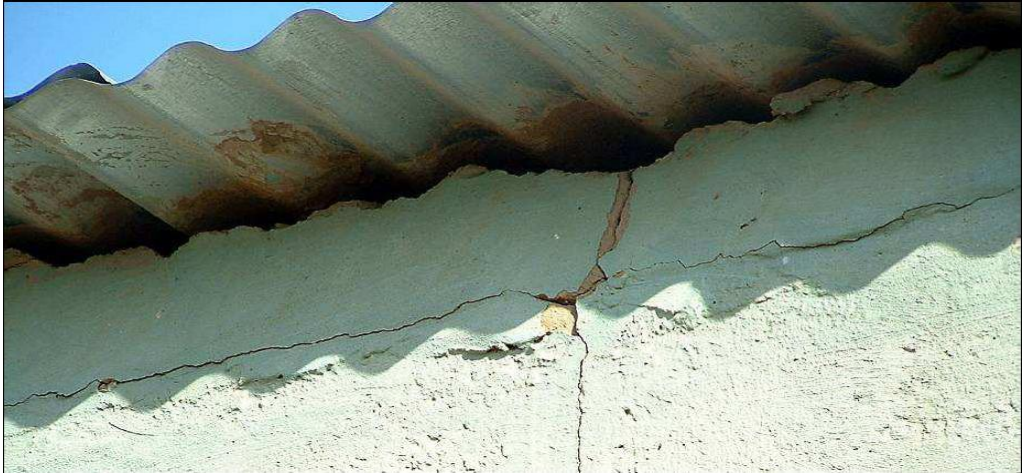
Figure 4: Cracked Wall and Unsecured Roof. Peddie, Eastern Cape. Source: de Nobrega, 2007: 11.
