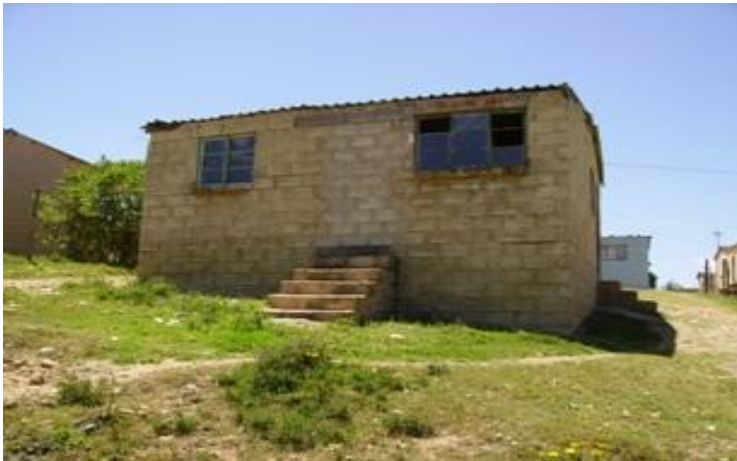
Figure 2: Construction Error. Hankey, Eastern Cape. Source: Khanya-aicdd, 2008: 10.
