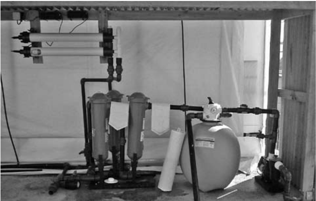
Figure 34. Seawater filtration system.
