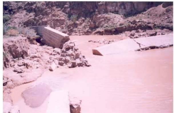
Fig-4 Failed Side intake constructed on Bilate River
