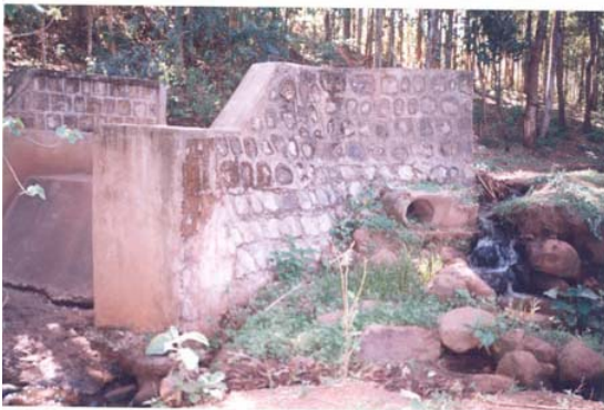
Fig-2 Failed Hao diversion weir
