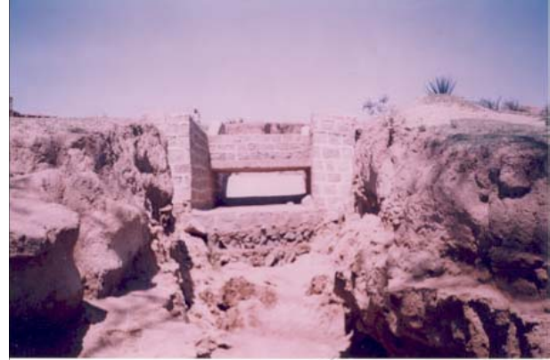
Fig-7 Scouring problem on an aqueduct at Lenda Project
