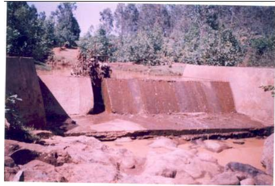
Fig-5 Failed Goche diversion weir
