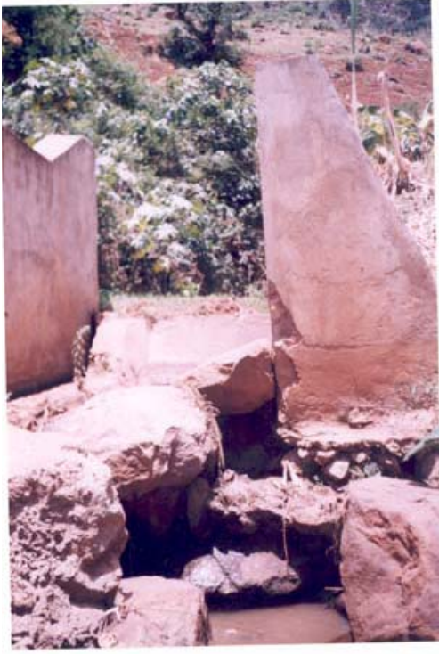
Fig-3 Failed Hazembara diversion weir
