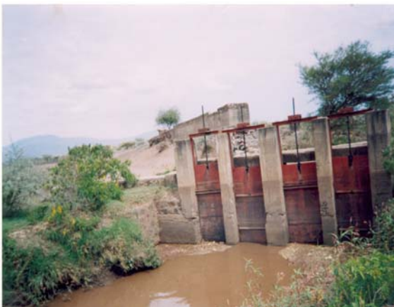
Main gate on the main canal at Nuraera
