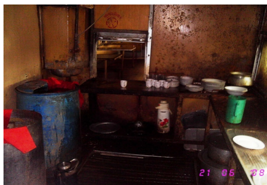
FIGURE 3: VERY UNHYGIENIC KITCHEN
