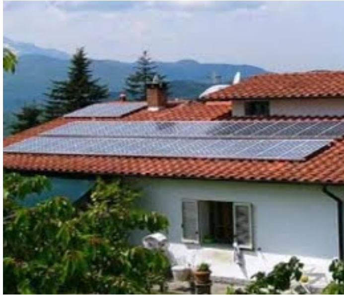
Figure 1: An installation of PV panels
