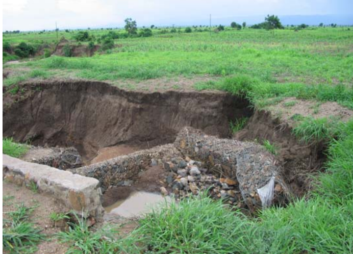
Figure 3.14: Landslide Gully Erosion during torrential rains causing severe damage to socio-economic structures in Mulanje - Phalombe areas
