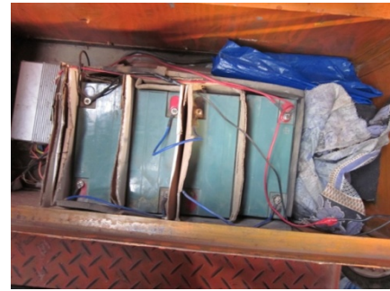
Fig.3.3 Batteries accommodated inside the seat
