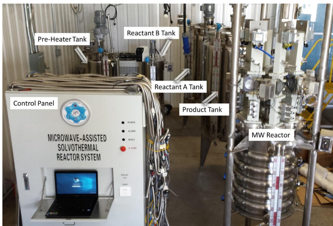
Figure 7-14. Commissioned MW reactor system
