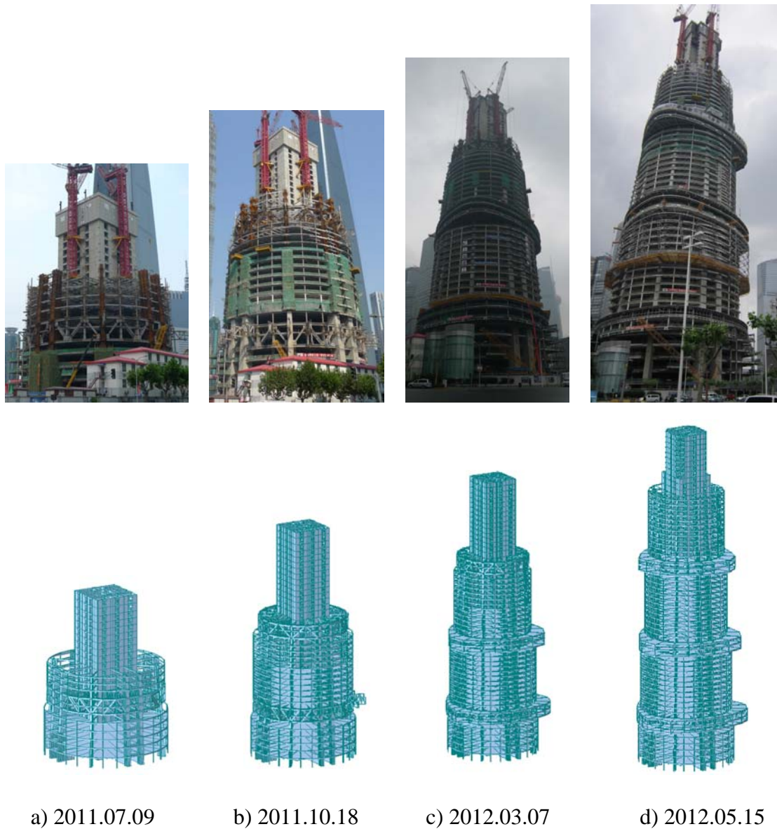
Fig. 8. Photographs of the Shanghai Tower and the corresponding FE models at different construction stages.
