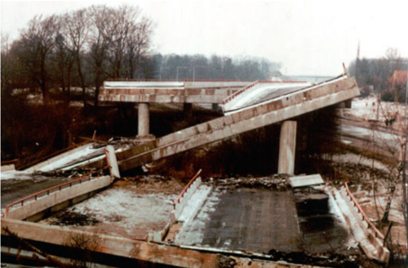
Fiskebækbroen collapsed 8 February 1972 before it had been taken into use. Source: The Danish Road Directory.
