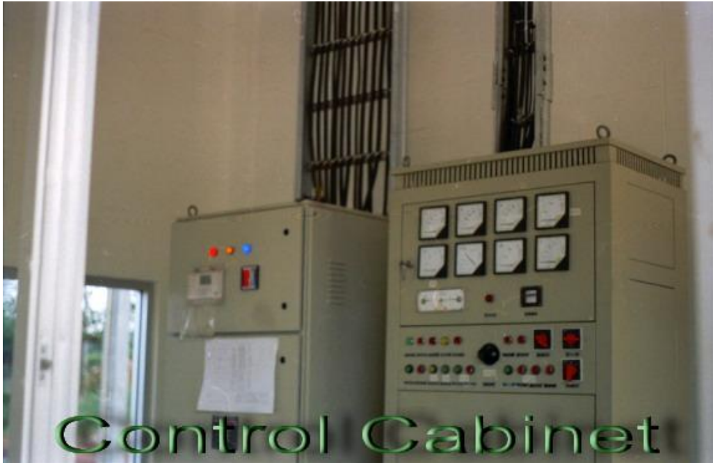
Figure A1-11: Control Cabinet
