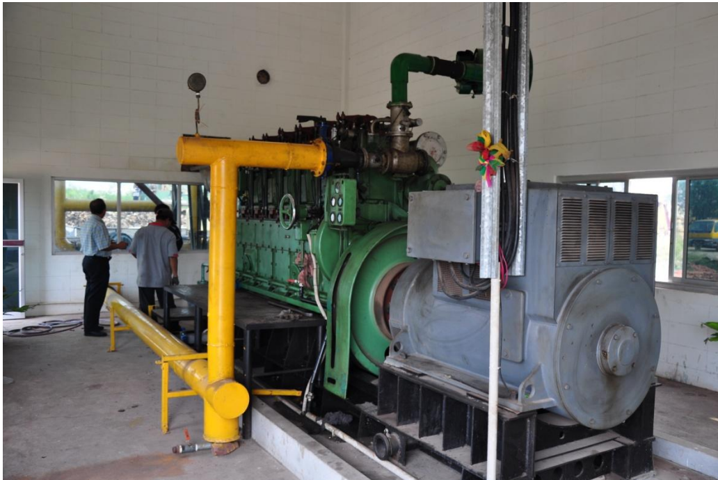
Figure A1-15: Gas Engine Generator
