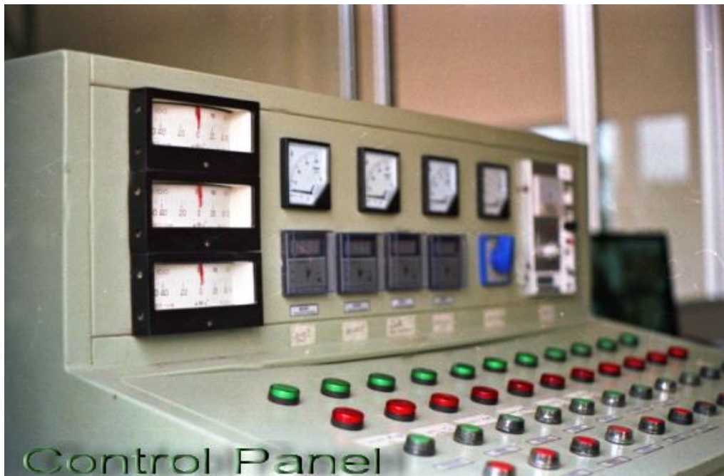
Figure A1-10: Control Panel
