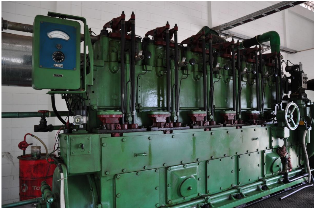
Figure A1-16: Gas Engine Generator with 6 Cylinders
