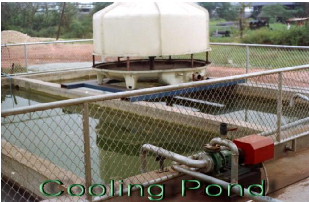
Figure A1-14: Cooling Pond
