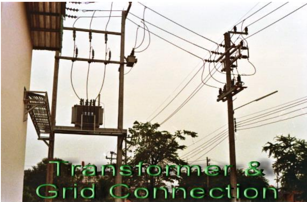
Figure A1-12: Transformer & Grid Connection
