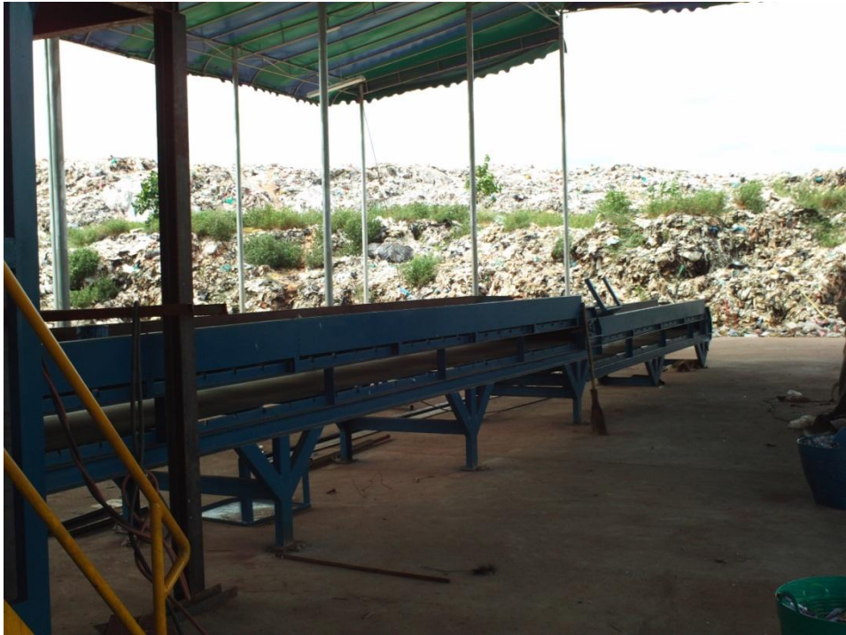
Figure A1-5: Large size waste (RDF) conveyor after screen
