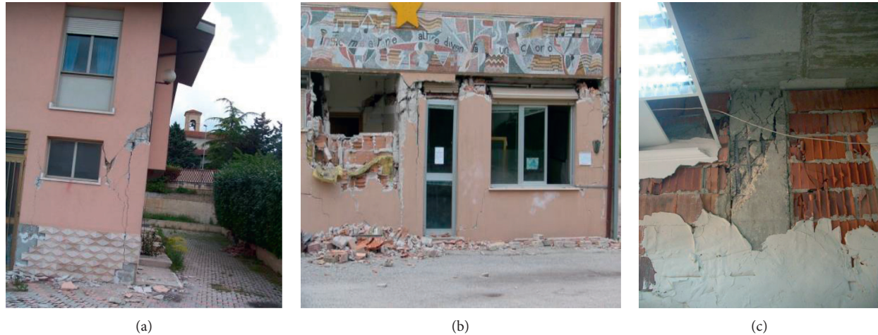
FIGURE 4: Example of in-plane shear interaction between infill panels and RC frames adapted from [7, 24]. (a) L'Aquila (2009). (b) L'Aquila (2009). (c) Lorca (2011).
