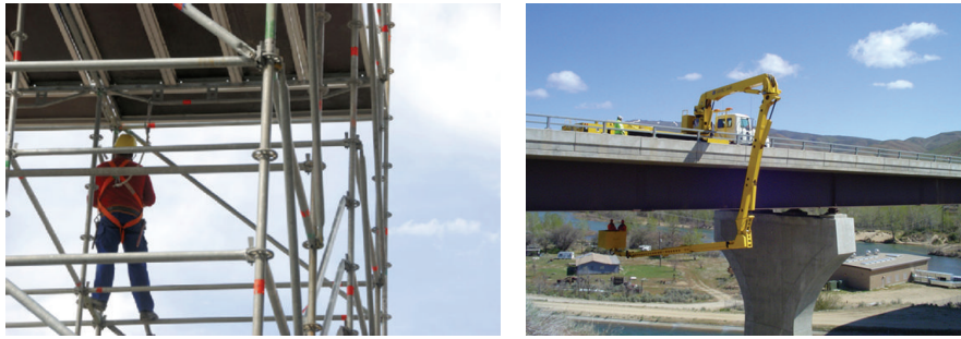
FIGURE 3: Two common ways to inspect bridges: scaffold and inspection truck with crane.
