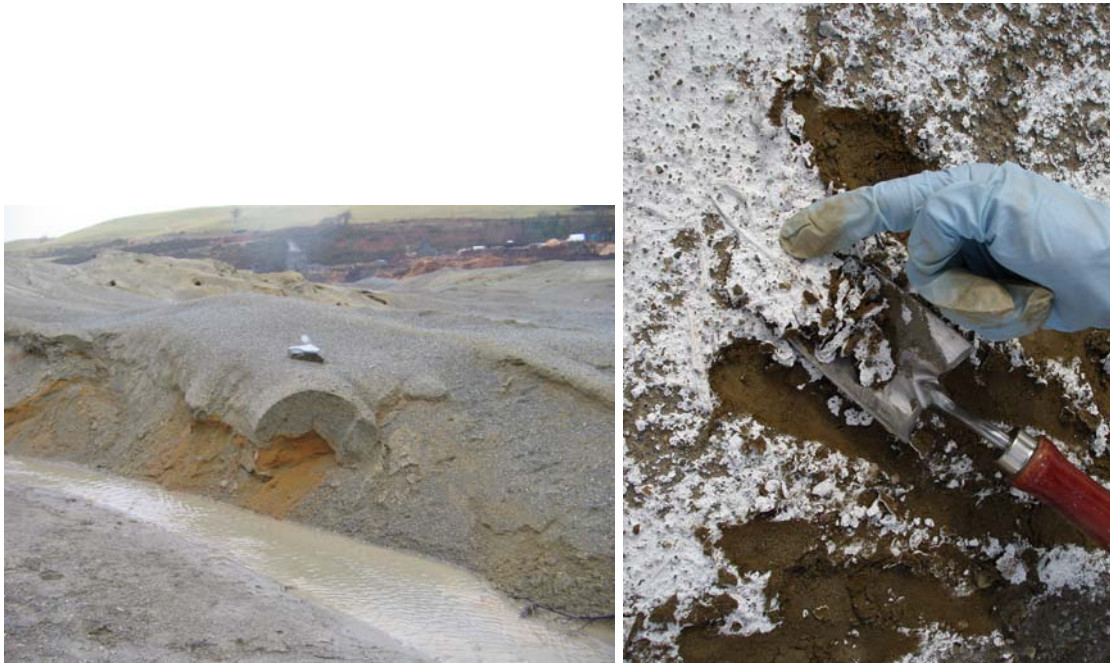
Figure 5: Channelling in the tailings. Figure 6: Bianchite on tailings, August 2006.
