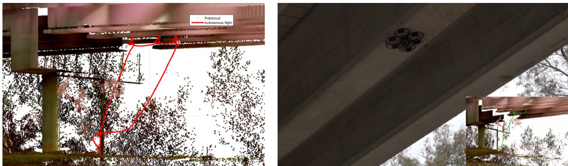
Figure 1.4: UAV measuring beam deflection in a bridge. Left, UAV trajectory during the mission with a point-cloud captured by the Total Station. Right, snapshot of the UAV stuck to the beam.
