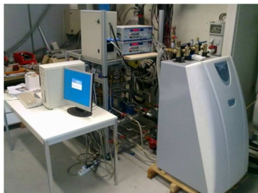
Heat pump module connected to a heat pump
