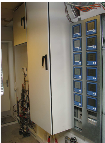
Heat meters at EnergyFlexLab.
