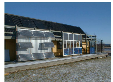
Test of pv systems.
