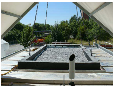
ILARGI: installing the roof covered by gravel to be tested inside the frame.
