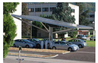
Electrical cars and solar station.
