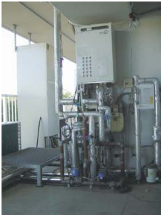
Boilers and CO 2 heat pump system for DHW: Efficiency of several heat sources is measured with changing connection between the heat source and piping dwelling unit.
