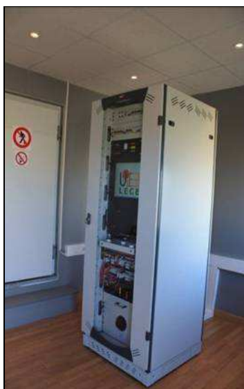
Rack mounted computer and data acquisition system in the service room of a test cell.
