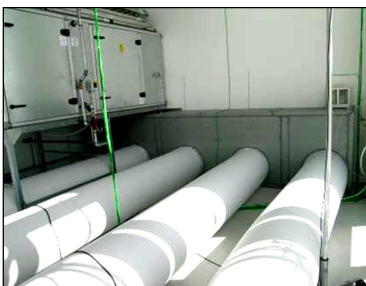
KE-low impulse fabric ducts in the experiment room
