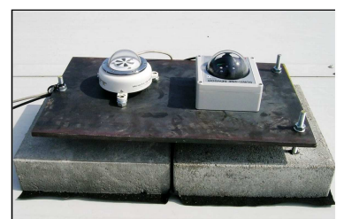
Photo of pyranometers on the roof of the Cube, Wilhelm Lambrecht pyranometer at the left and BF3 at the right
