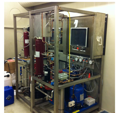
Test of heat pumps.
