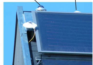
Pyranometers and pyrgometer at the roof of EnergyFlexLab.
