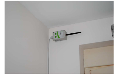
Sample sensor used for measuring temperature and humidity levels throughout the house.
