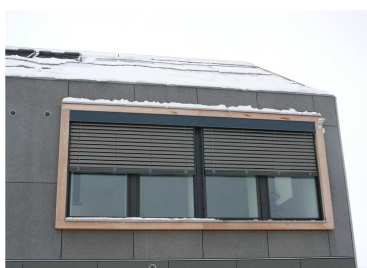
Sun screening of the windows facing south on EnergyFlexHouse.
