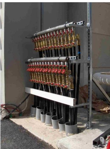
Manifolds connected to the ground heat exchangers
