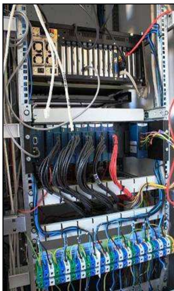
Data acquisition system in the service room of a test cell.
