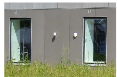
Pyranometer and temperature sensor at the south wall of EnergyFlexLab.
