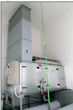
Ventilation system in the experiment room
