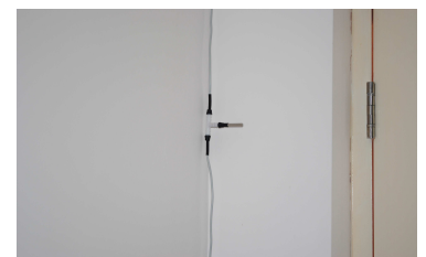
Sample temperature probe used within the Energy House.
