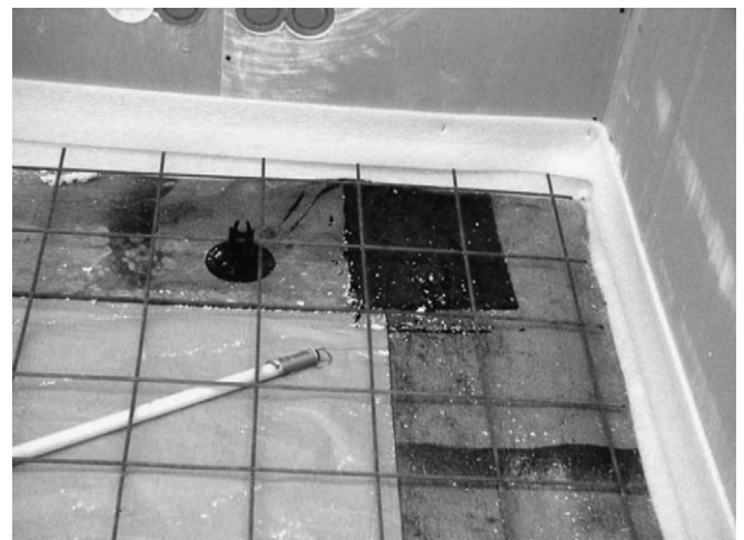
Fig. 3. Bitumen felt installed to the joint of foundation wall and floor slab before casting of the floor [34].
