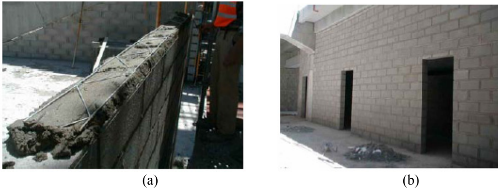
Figure 2 Sporting Club Stadium, Portugal: (a) implementation of bed joint reinforcement, (b) the final appearance of walls [4].
