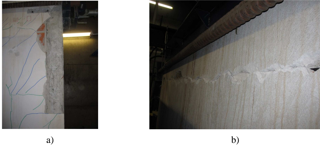
Figure 19: In-plane apparent state of damage: a) lateral interface; b) upper interface
