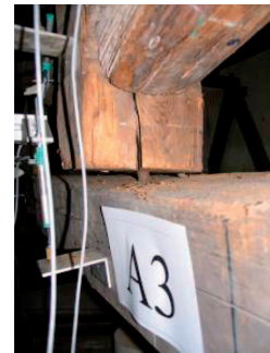
Figure 12. Out-of-plane movement observed in the truss 1 (unstrengthened) under ULS at the end of 1st cycle.
