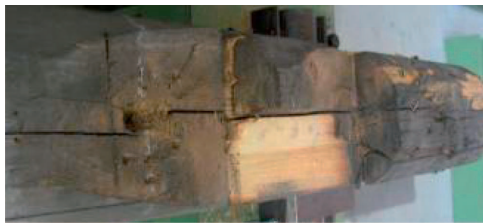
Figure 16. Shear failure of the rafter/tie beam connection for Truss 2.
