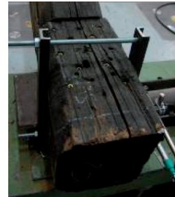
Figure 14. Strengthening of Truss 2. Screws and binding strip applied in the frontal part of the step in the rafter/tie beam connection.
