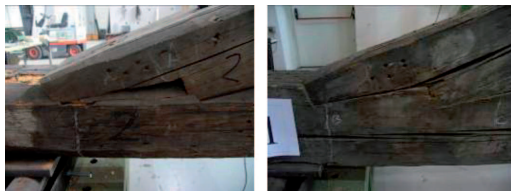
Figure 17. Double step connections between the rafters and the tie beam of Truss 2.
