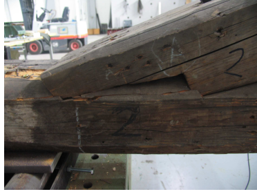
(a) Failed (right side)
