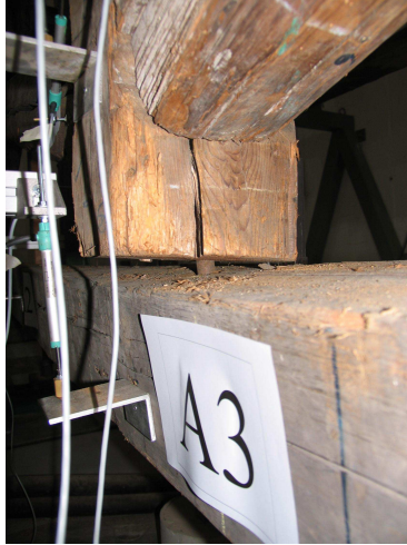
Figure 14: Out-of-plane movement observed in the Truss 1 (unstrengthened) under ULS at the end of 1 st cycle.
