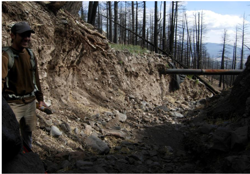
Figure 4. Deeply incised (3 m) main drainage gully within the Schultz Fire along the Waterline Road, Coconino National Forest, Arizona.
