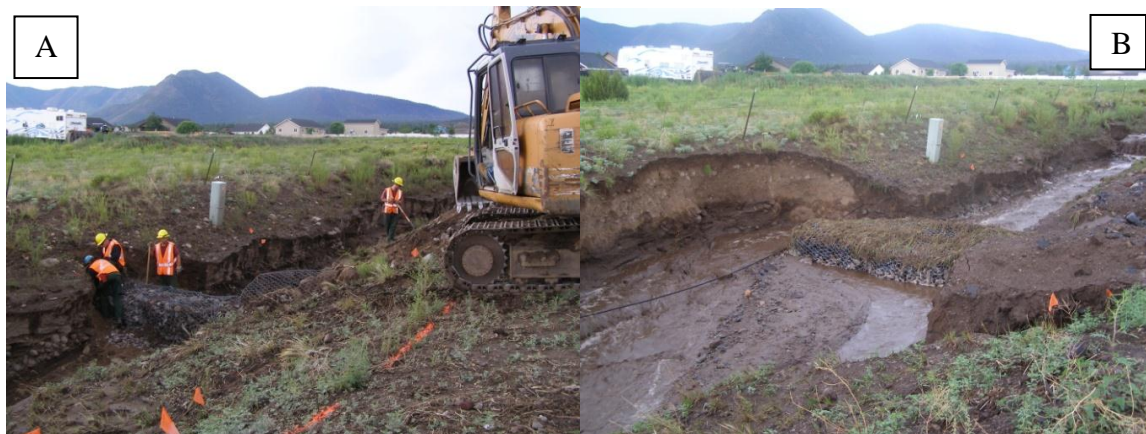
Figure 3. Gabion construction along Campbell Avenue prior to the July 30, 2010, storm (A); and results during the storm event showing gabion failure and channel widening (B).
