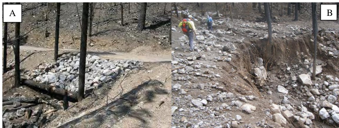
Figure 1. Rock armoring along the Waterline Road before (A) and after (B) the July 20 th flood.
