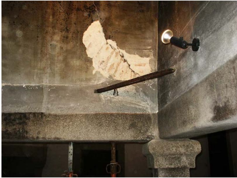
Figure 3 – Typical aspect of an inspection opening to uncover the internal arching system
