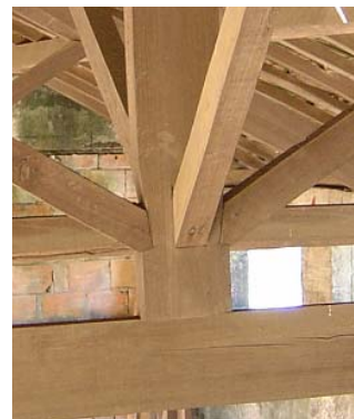
Fig 7 Example of a misconceived connection between the king post and the tie-beam
