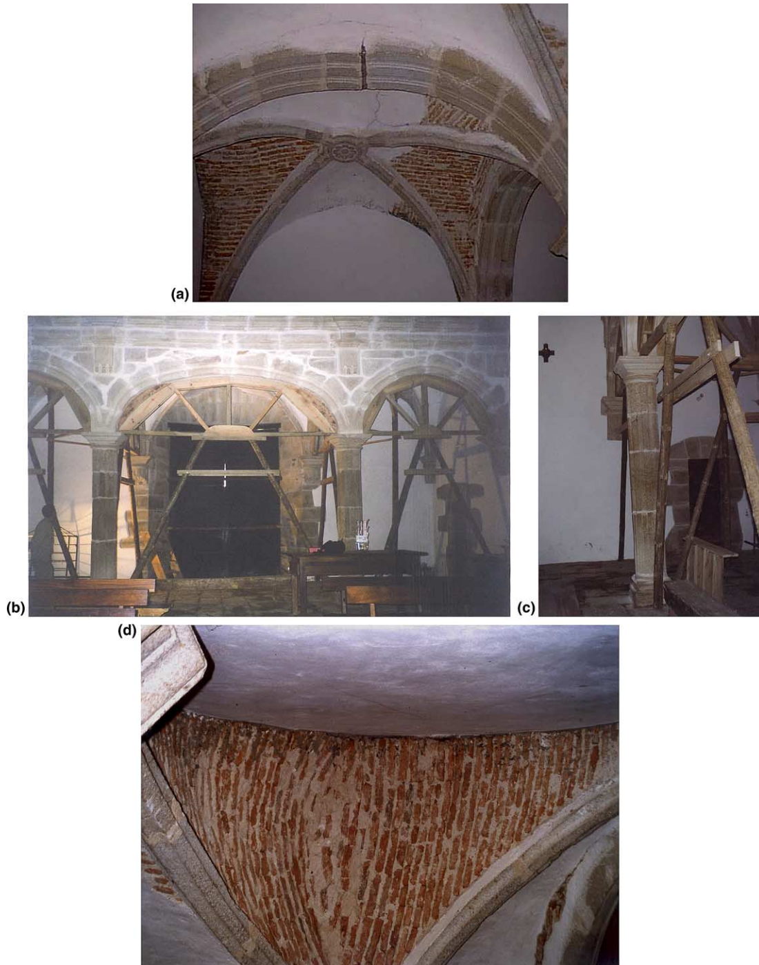
Fig. 5. Aspects of the damage in the choir: (a) cracked ribs; (b) temporary support; (c) columns out-of-plumb; (d) no connection between vaults and walls.
