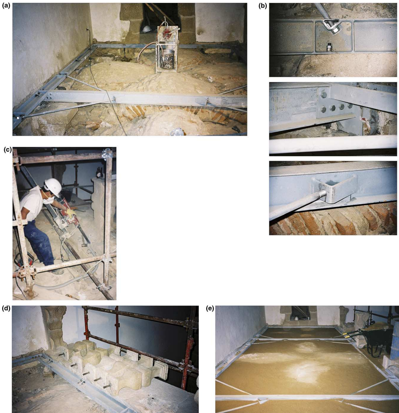
Fig. 13. Aspects of the execution: (a) general view of the steel frame, tie and injection of the vaults; (b) details of the steelwork; (c) drilling of the holes for the anchors; (d) aspect of the dowels used in the balusters; (e) final aspect of the vault, with the soil infill.
