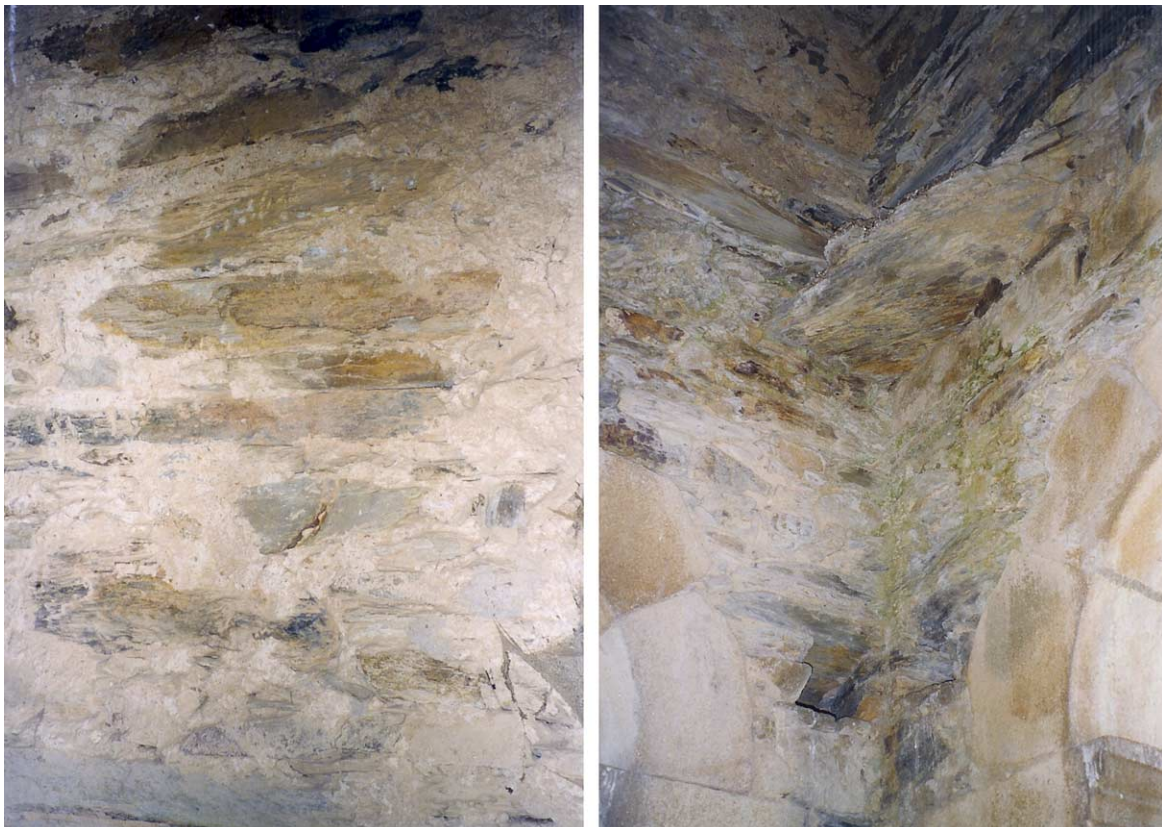
Fig. 1. Aspects of the irregular masonry in non-plastered areas, including ashlar around window openings.
