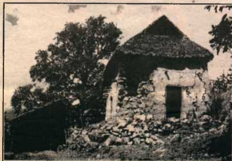
courtesy of MSNBC Common structure damage of stone homes in an Earthquake
