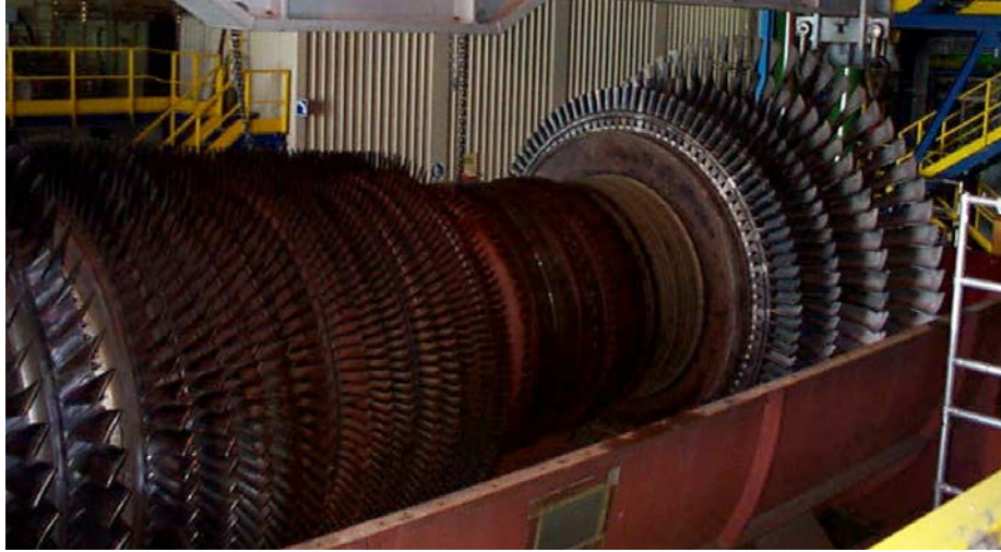
Figure 22: Close up of the compressor and turbine of the considered gas turbo-generator.
