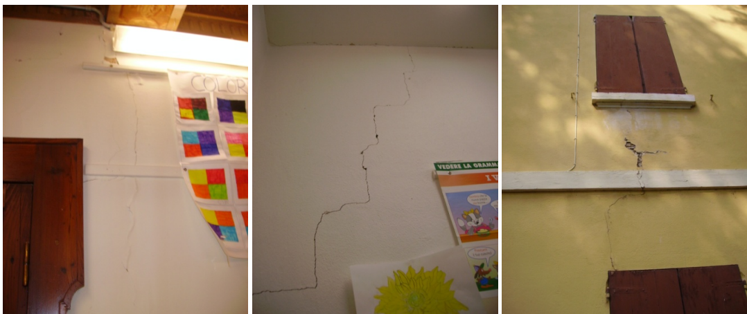
Figure 6: Details of some internal and external cracks.
