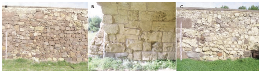
Figure 4. Sequence of the masonries concerning the south façade: A) part near the first arches towards west; B) detail of the interior of one of the arches; C) the terminal part towards east.
