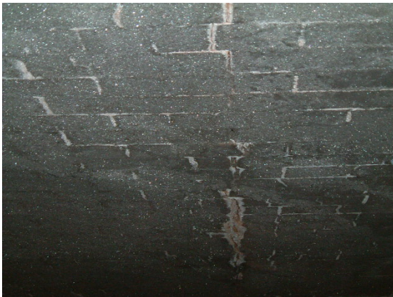
Figure 4: Typical cracks along a flue wall
