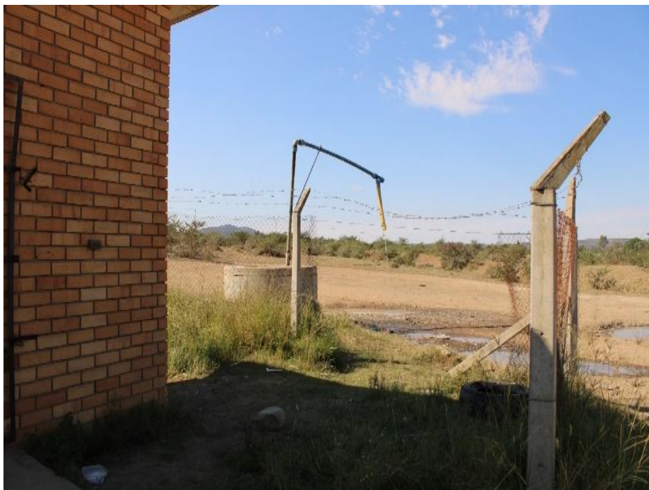
Figure 0.4: Leaking communal pipe in Amathole Water treatment plant
