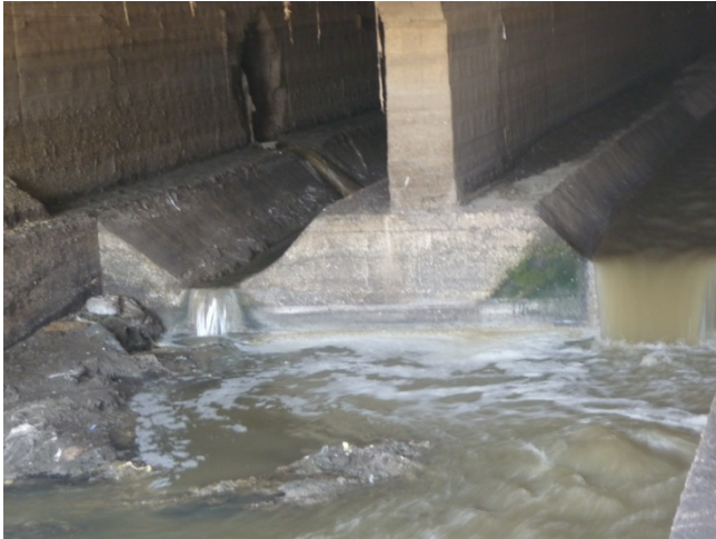
Figure 2: Example of deposit in a CSO chamber.
