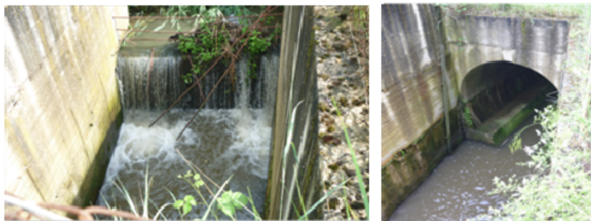
Figure 3: Cesarina stream – inlet to combined sewer.
