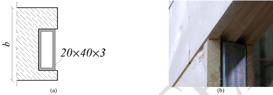
Fig.4. Steel hollow profiles introduced along the vertical edges of openings (specimens W03 and W04). (a) Nominal cross-section, dimensions in mm; (b) detail near the top corners of the door opening.
